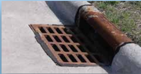
Storm Drain / Catch Basin
