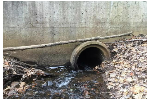
Image 1: Existing structure inlet during field visit on November 25, 2020. Note the inlet drop and misalignment of the stream with the inlet.
