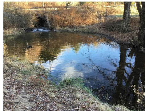
Image 2: Existing structure outlet during field visit on November 24, 2020. Note the large scour pool, eroded banks, and perched outlet.
