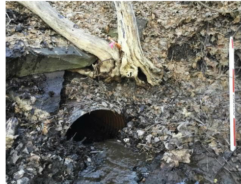
Image 1: Existing structure inlet during field visit on December 4, 2020, showing a blockage causing a drop into the inlet and erosion on the bank above the pipe.
