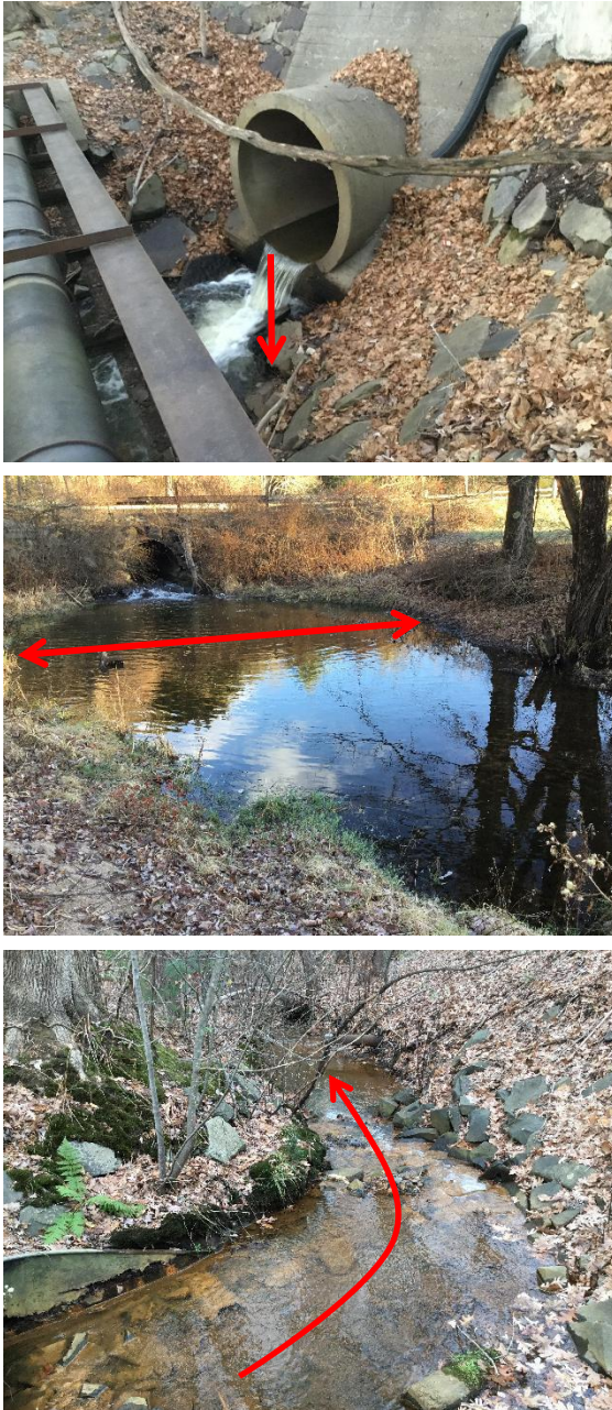
Figure 8. Geomorphic Vulnerability Ratings/Scores consider factors such as outlet drops which contribute to scour, the bankfull width of the stream, and alignment of the stream with the structure. The Main Street crossing over Buttery Brook (top) received a Geomorphic Vulnerability Score of 4 due to the free fall at the outlet as well as flow constriction and alignment factors. The Pearl Street crossing over Elmer Brook (middle) has a very wide tailwater scour pool at the outlet. The Willimansett Street crossing over Buttery Brook (bottom), where the stream bends immediately after leaving the outlet, demonstrates poor alignment of the crossing structure with the stream.
