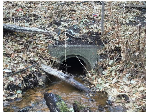
Image 1: Existing structure inlet during field visit on November 25, 2020, showing a blockage causing a drop into the inlet and erosion of the banks to either side.
