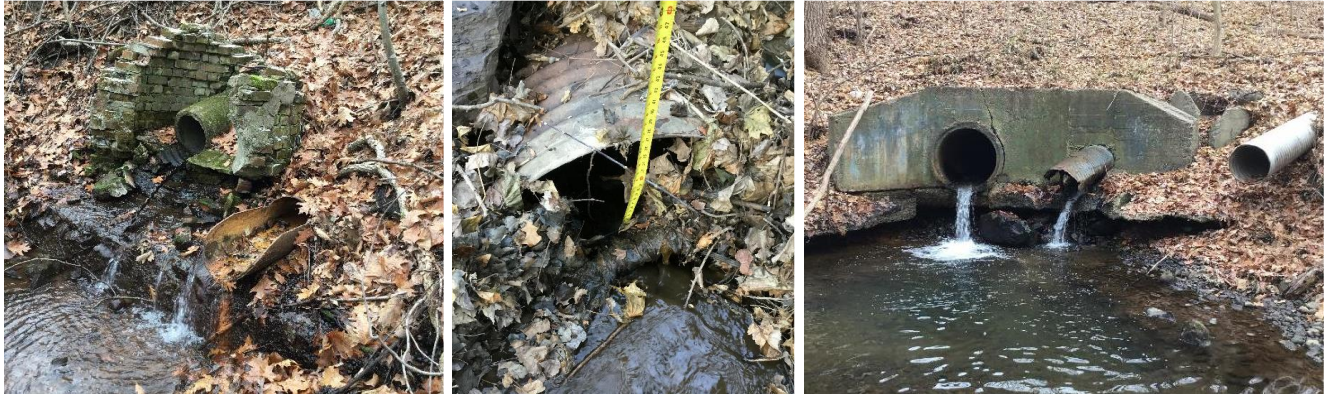
Figure 3. Examples of crossing structures in poor structural condition observed at various locations during field assessments.
