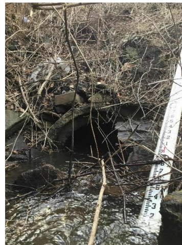
Image 2: Existing Brainerd Street culvert inlet during field visit on December 10, 2020.
