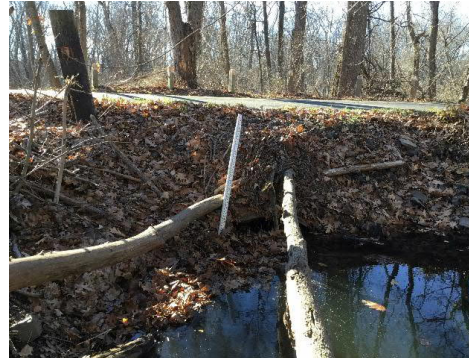
Image 1: Existing structure inlet during field visit on December 10, 2020, showing only the top of the pipe. The rest of the inlet is buried under sediment and debris.
