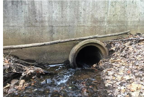
Image 1: Existing structure inlet during field visit on November 25, 2020. Note the inlet drop and misalignment of the stream with the inlet.
