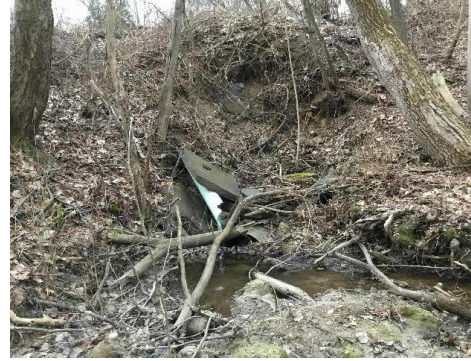
Image 1: Existing structure inlet during field visit on December 9, 2020, showing a blockage at the inlet and the collapsed bank above the pipe.
