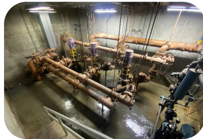
Return/Waste Activated Sludge & Scum Pumps
