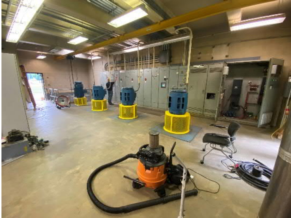
Main Street Pump Station 4 th Floor: Four (4) Vertical Dry Pit Pump Motors.
