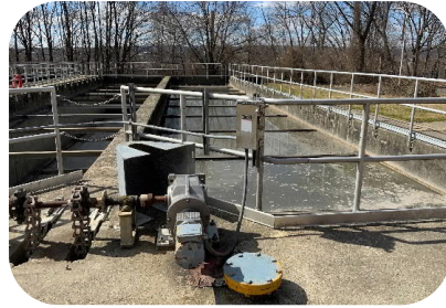
Primary Clarifier Sludge Collectors
