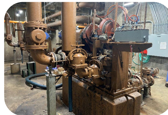
Primary Sludge Pumps
