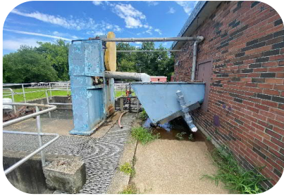
Gravity Bucket Elevator
